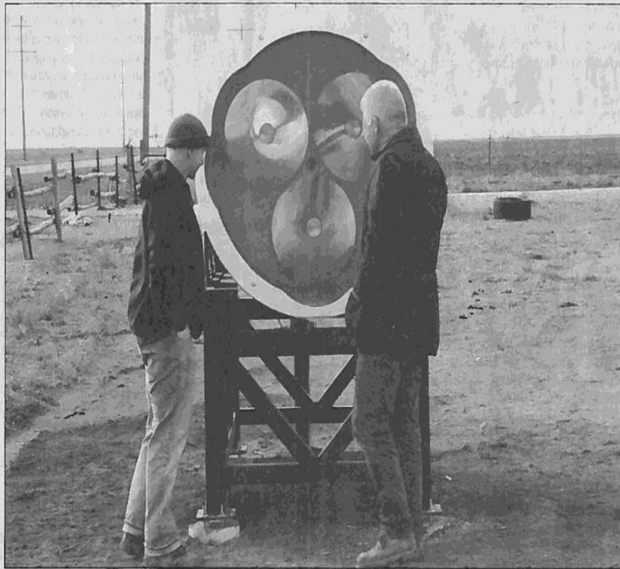
Steve Plowman, a representative of the MIDAC Corp., left, and Ken Casey, Texas AgriLife Research air quality engineer, check the installation of the infra-red light source.
